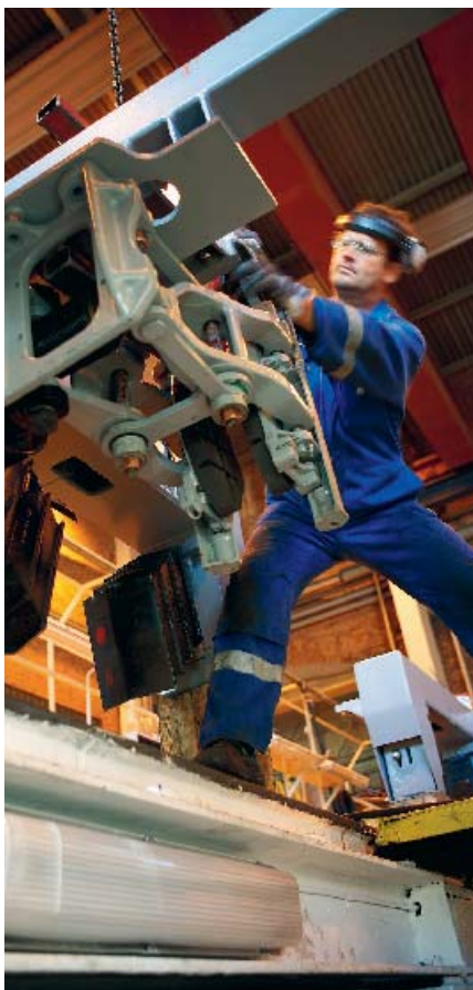
EuroMaint offers qualified maintenance which increases the service life of customers' production equipment.
